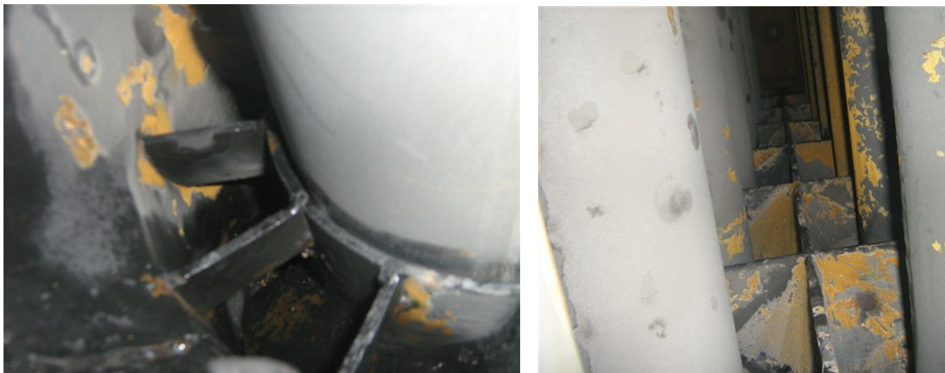
GRIT ARRESTORS BEFORE CLEANING
